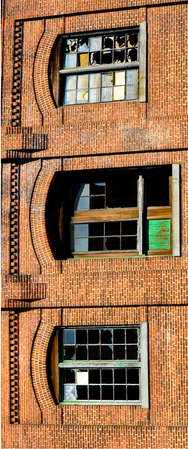
Figure 43: Detail of window damage common to the site (photo by author).
