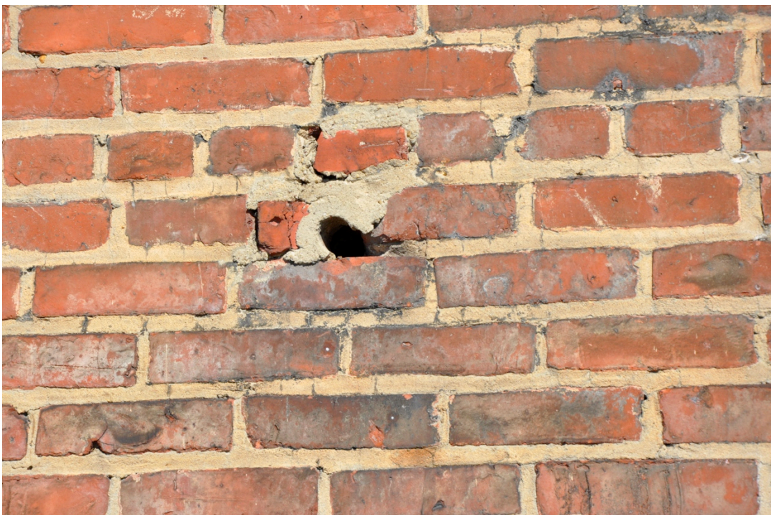
Figure 46: Detail of improperly treated brick (photo by author).
