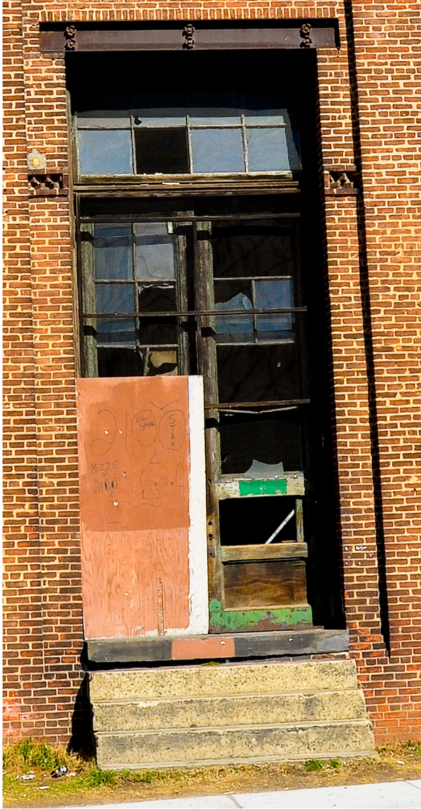
Figure 44: Detail of damaged front entrance, (photo by author).
