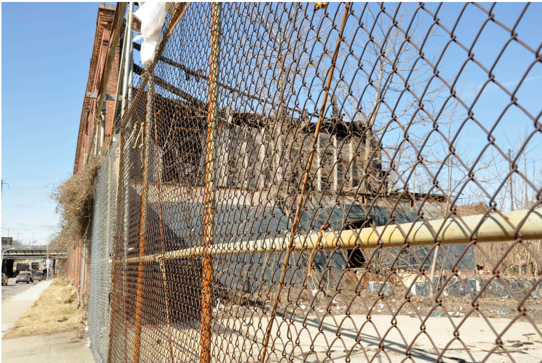
Figure 40: Detail of fire damage to eastern wall of the tank house (photo by author).
