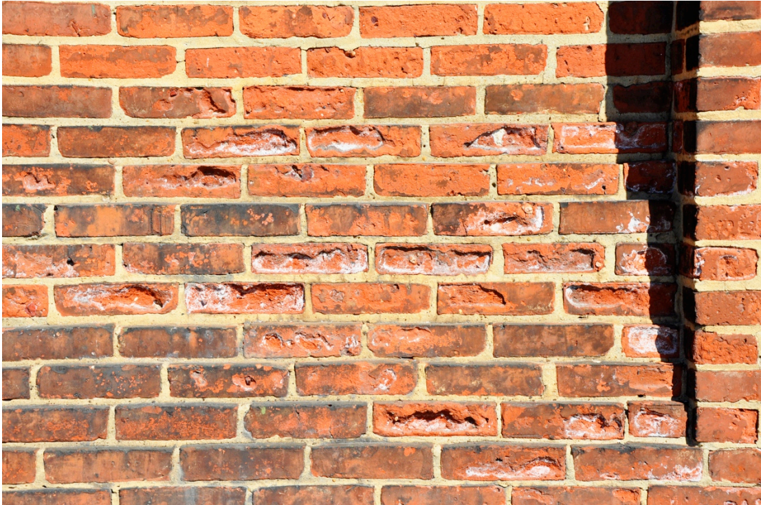
Figure 45: Detail of brick spalling (photo by author).
