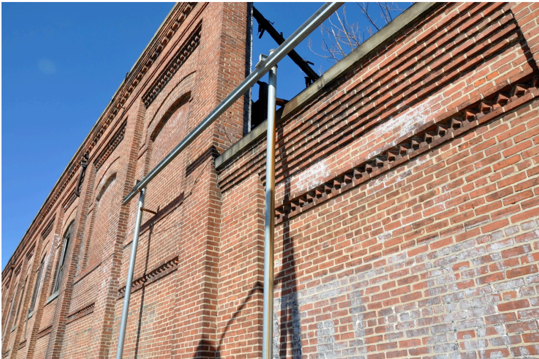
Figure 48: Intact tracking for gate (photo by author).
