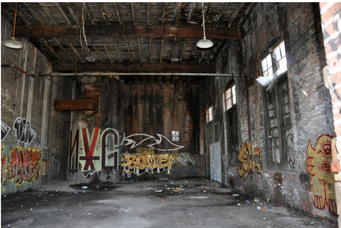
Figure 42: Interior of boiler and engine room (photo by author).
