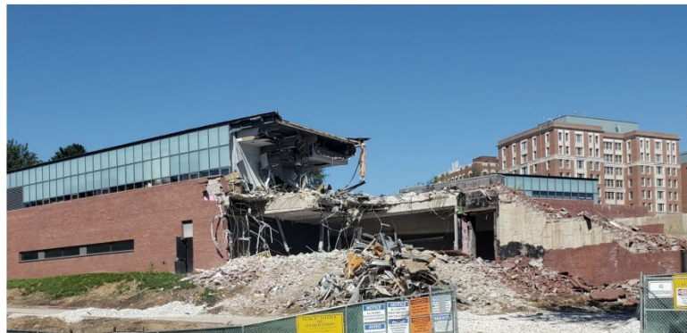
Figure 3: Demolition of the Mattin Center at Johns Hopkins University began in 2021, just 20 years after its completion. (Ed Gunts, Baltimore Fishbowl)
