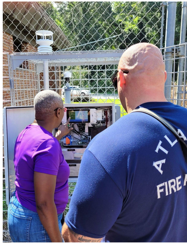
D. Powering on AQSunc in Collier Heights
