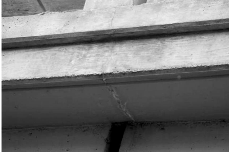
Figure 2-6 Full-depth crack in link slab that was observed in the inspection (Ulku et al. 2009)
