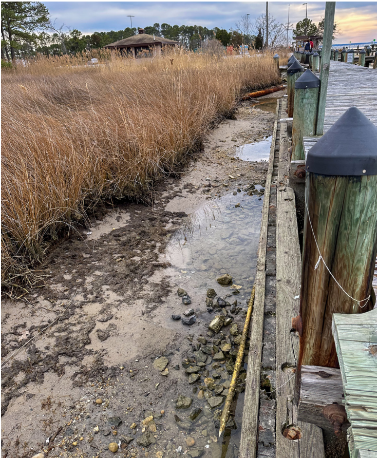
Figure 71: Eroded shoreline behind existing dock
