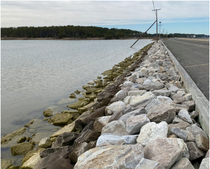
Figure 63: Revetments along the Chesapeake Bay side
