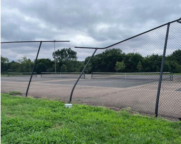
Figure 93: Damaged fence in tennis courts. Credit: the author.
