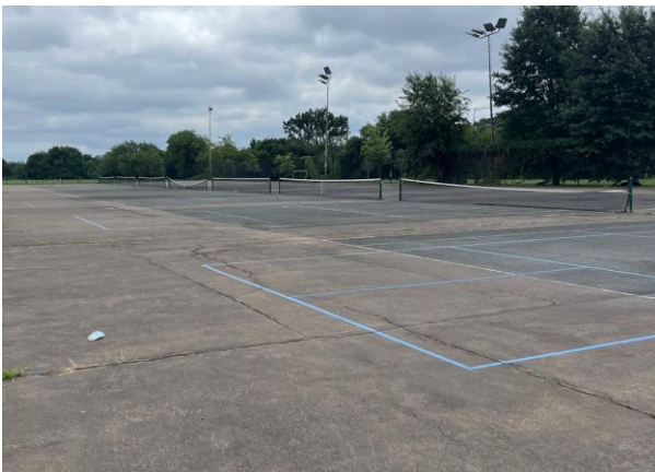
Figure 95: Tennis Courts in Neglected Conditions. Credit: the author.
