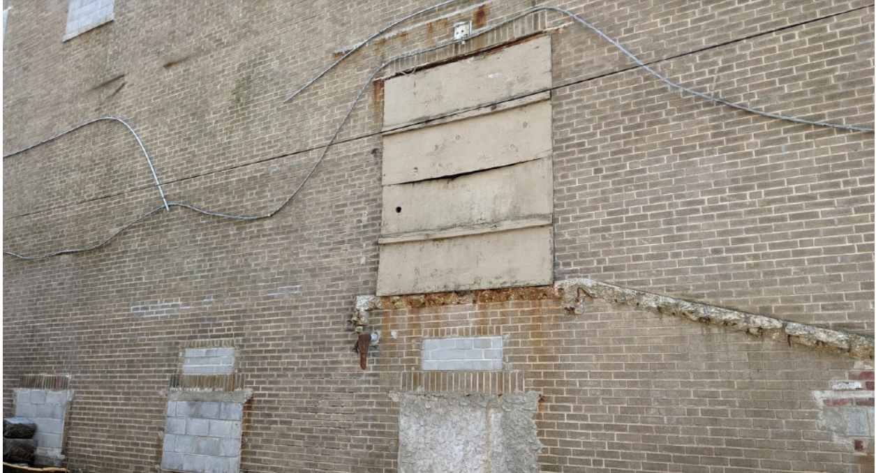
Fig. 21: Evidence of permanent infill; the outline of concrete reinforced service ramp; rust present where reinforcing bars were once present, March 2022 (Source: Author)
