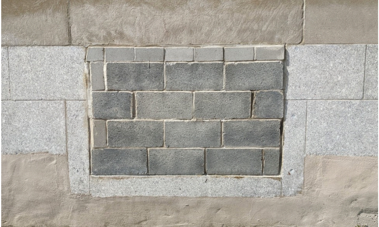
Fig. 10: The granite water table has been repaired with incompatible concrete patchwork; windows have been permanently infilled with concrete masonry units; repair to mortar joints is inconsistent in profile, March 2022 (Source: Author)
