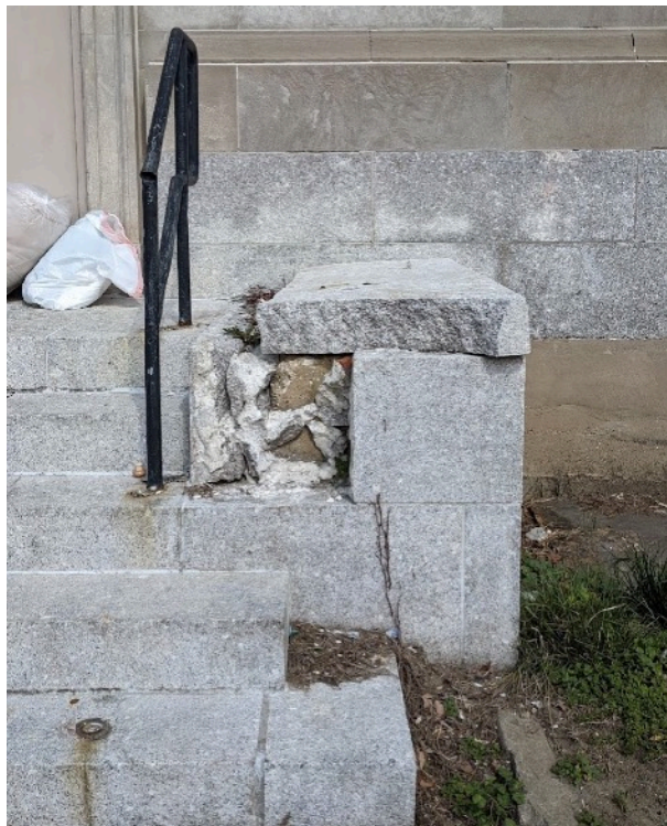
Fig. 16b: Severe deterioration of the granite entry steps reveals a rubble base, March 2022 (Source: Author)
