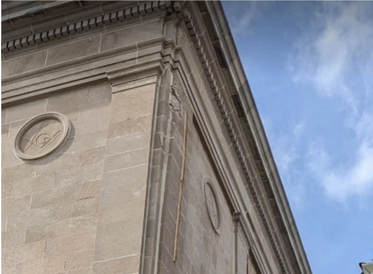
Fig. 24: Signs of deterioration at the corner pilaster; biological growth on underside of upper cornice; Masonic Emblems remain intact, March 2022 (Source: Author)
