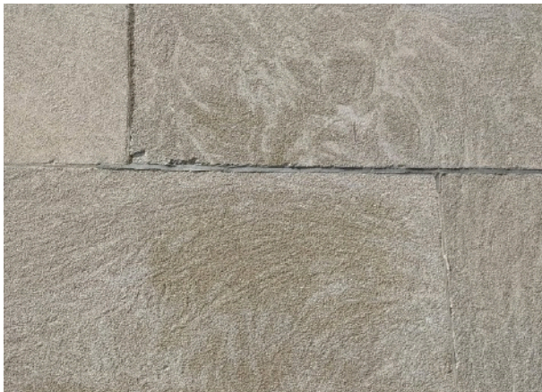
Fig. 12a: minor weathering of limestone faces; concrete mortar is causing spalling
