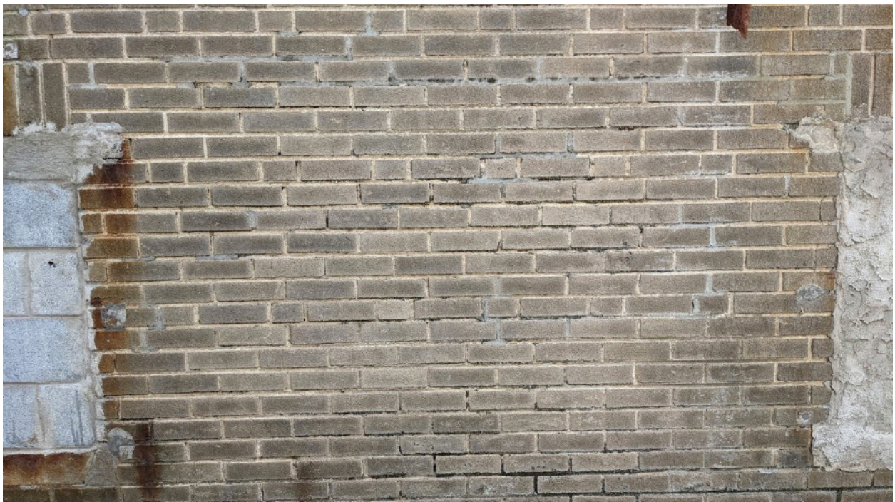
Fig. 22: Attempted mortar repair is visibly incompatible and high in cement content; mortar joints were not struck properly and show visible alteration in width; rust and concrete patchwork around basement windows indicates steel window grates were added and removed during period as a police precinct, March 2022 (Source: Author)
