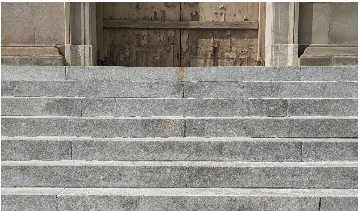
Fig. 11: The granite entry steps have minor rust staining due to previously installed metal handrails; minor spalling at joints; entry doors temporarily covered in plywood sheathing, March 2022 (Source: Author)
