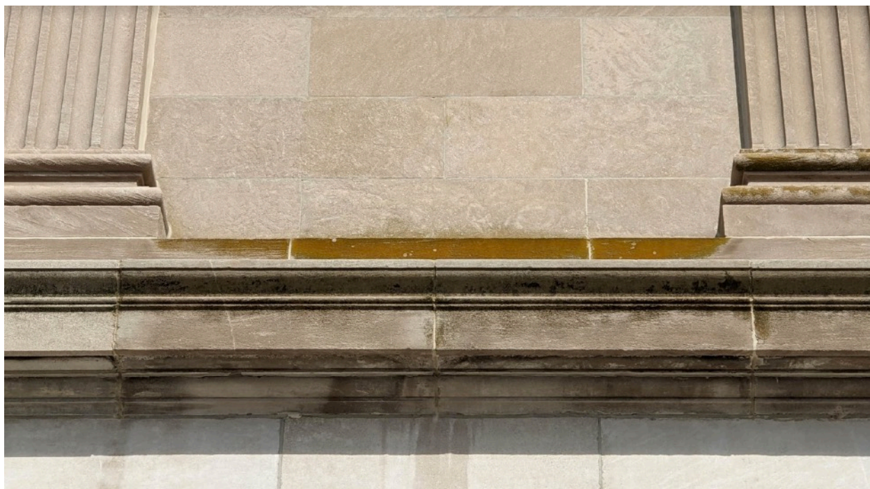
Fig. 17: Biological growth (black biofilm) on the shaded underside of the cornice; biological growth (algae based) on the cap of the cornice, March 2022 (Source: Author)
