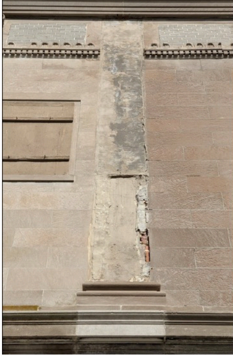
Fig. 18a: Missing pilaster exposes brick fill material, March 2022 (Source: Author)
