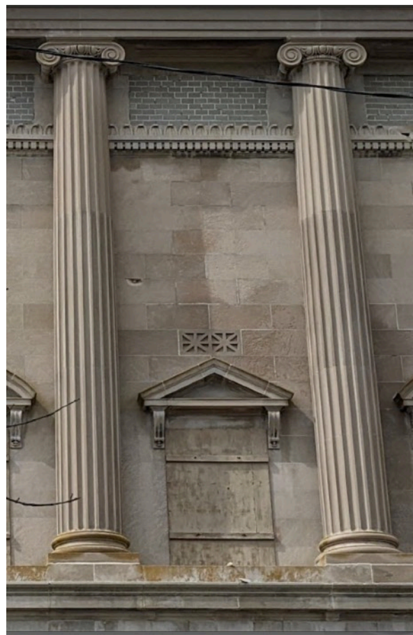
Fig. 13: Biological growth above and below cornice and aedicules; temporary protection of 2nd level windows; permanent infill of 4th level windows
