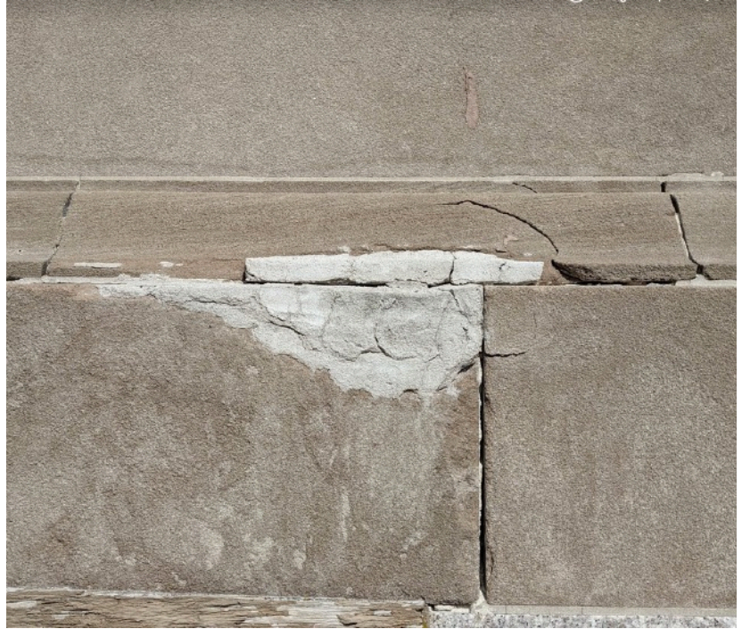
Fig. 18b: Severe spalling to the limestone due to concrete-based mortar repairs, March 2022 (Source: Author)
