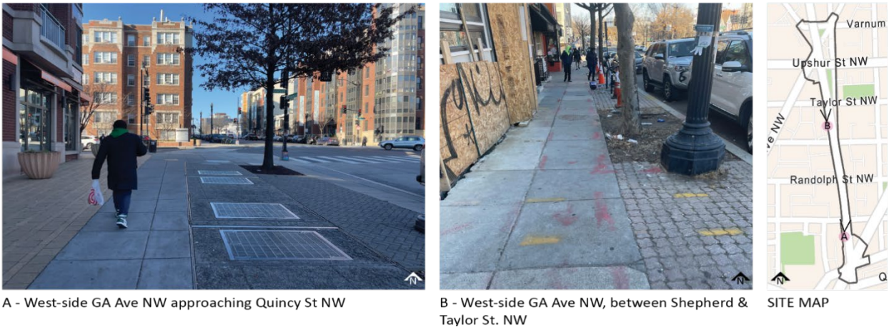
Fig. 3.15 Sidewalk conditions vary throughout the site, some areas are wide (A) and well maintained, others are degraded and barely meet minimum passage widths of 6 ft (B). Most do not meet the 10 ft commercial width requirement.
