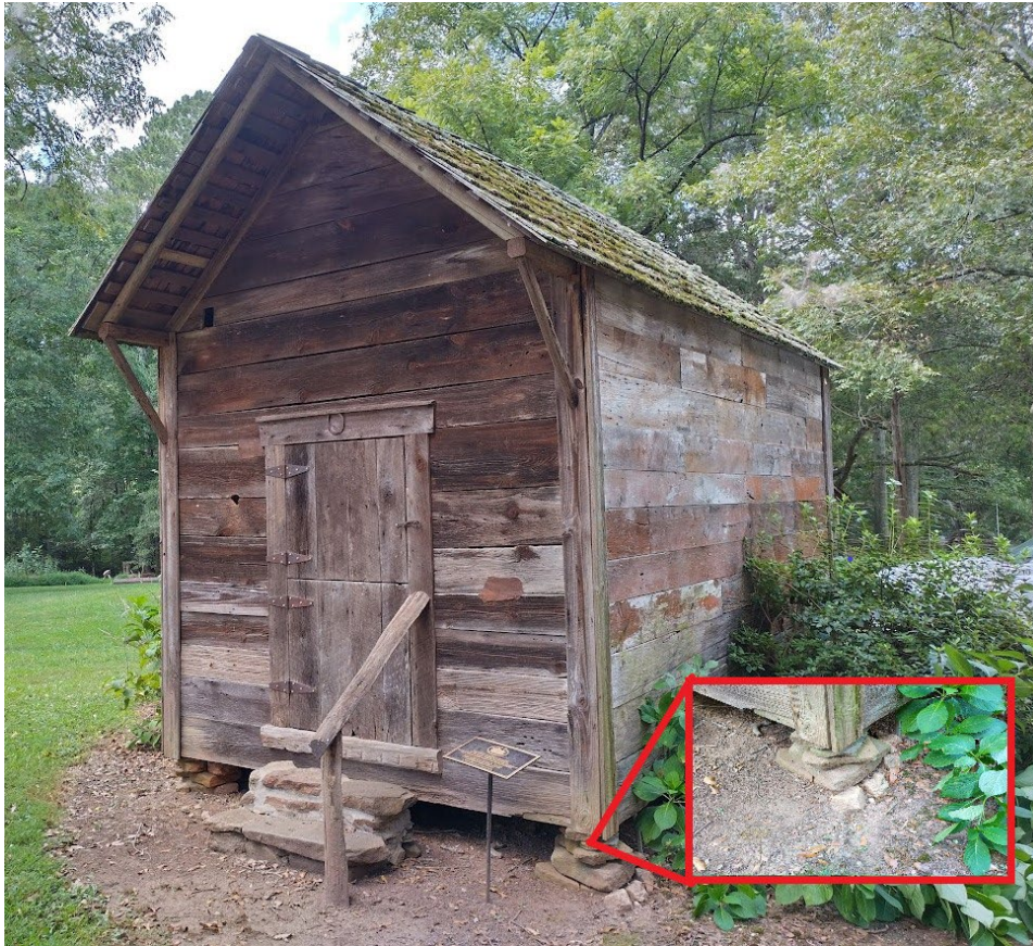
Figure 3.2. View of corn crib at 9WN168 and the stacked stone piers that support it, facing west (photo taken and edited by the author).
