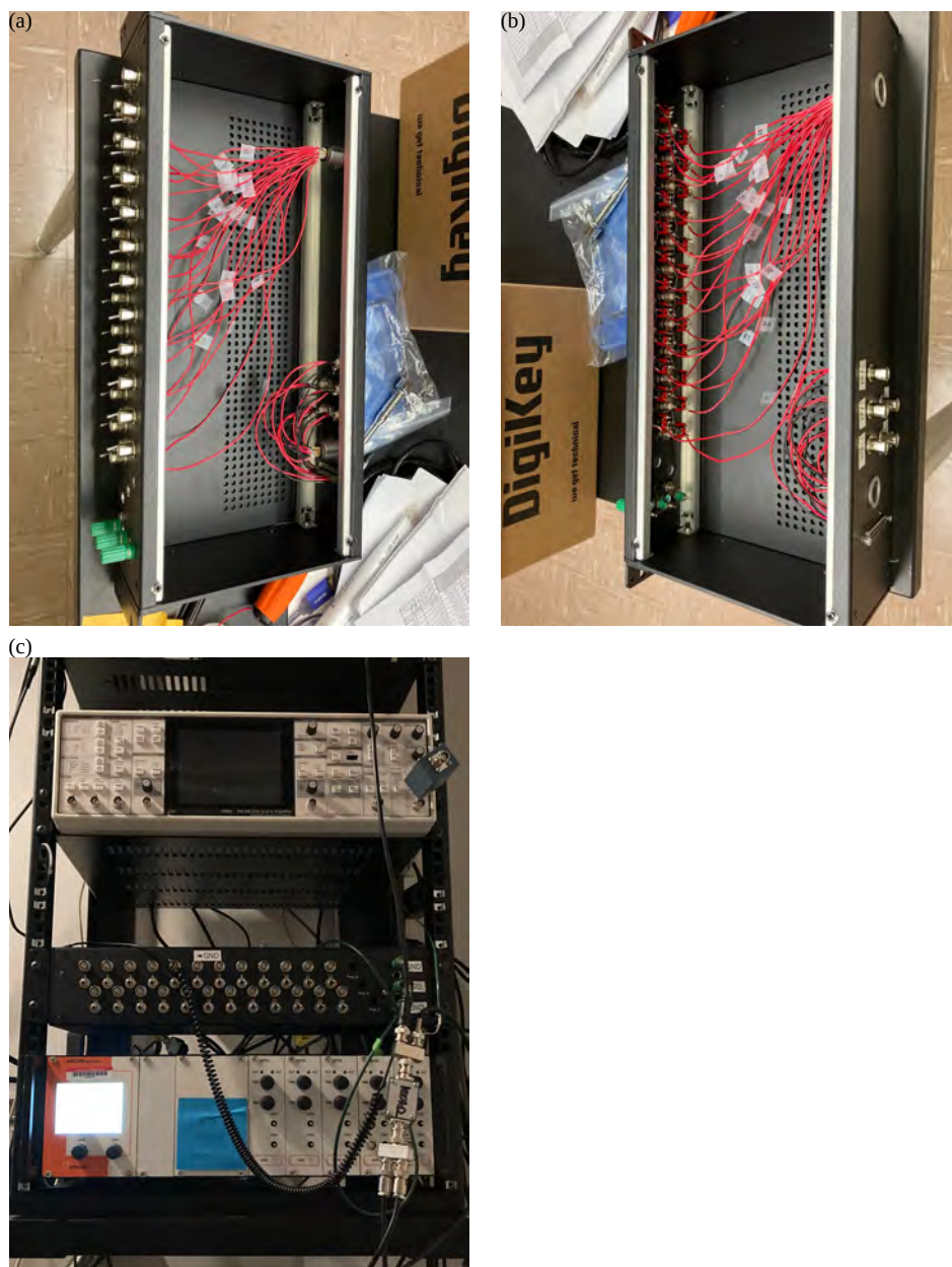
Figure C.1: Bluefors 2023 breakout box. Inside of the breakout box showing the wiring from the Fischer connectors to the BNC connectors for the Attocube lines (a), and the wiring for the BNC connectors for the DC lines (b). (c) The breakout box mounted on an electronics rack outside of the fridge.
