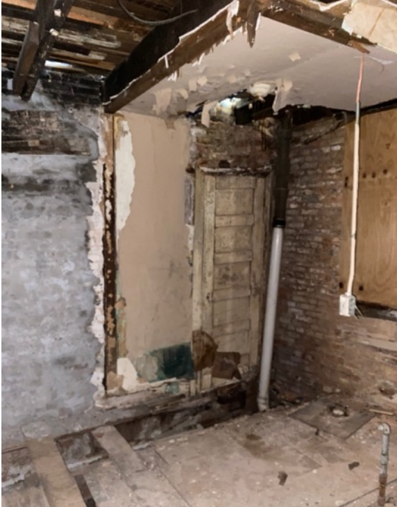
Fig.22, Sealed passage between the residential and commercial space, November 2022 (photo from author)
