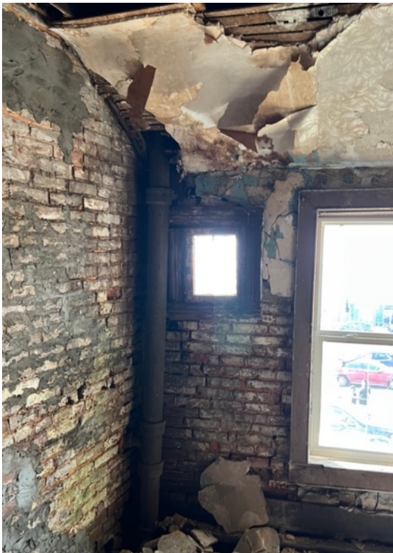
Fig.23, Second floor interior, rear portion of building, with wall finishes peeling off, November 2022 (photo by author)
