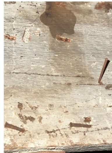
Fig. 15, Pre-1890 cut nails in wood beam, December, 2022 (Source: photo by author)
