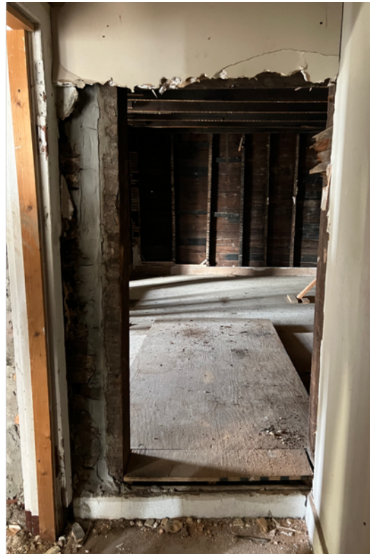
Fig. 24, Second floor of 1114 W. 36th St. with doorway having been carved out of existing brick wall in foreground; exposed wood stud wall on rear of the property in background, 2022 (photo from author)
