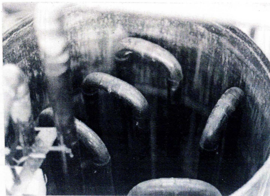
Figure 21 Inside Views of the Cooling System
