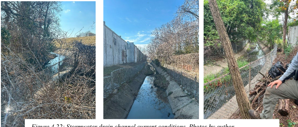
Figure 4.22: Stormwater drain channel current conditions. Photos by author.
