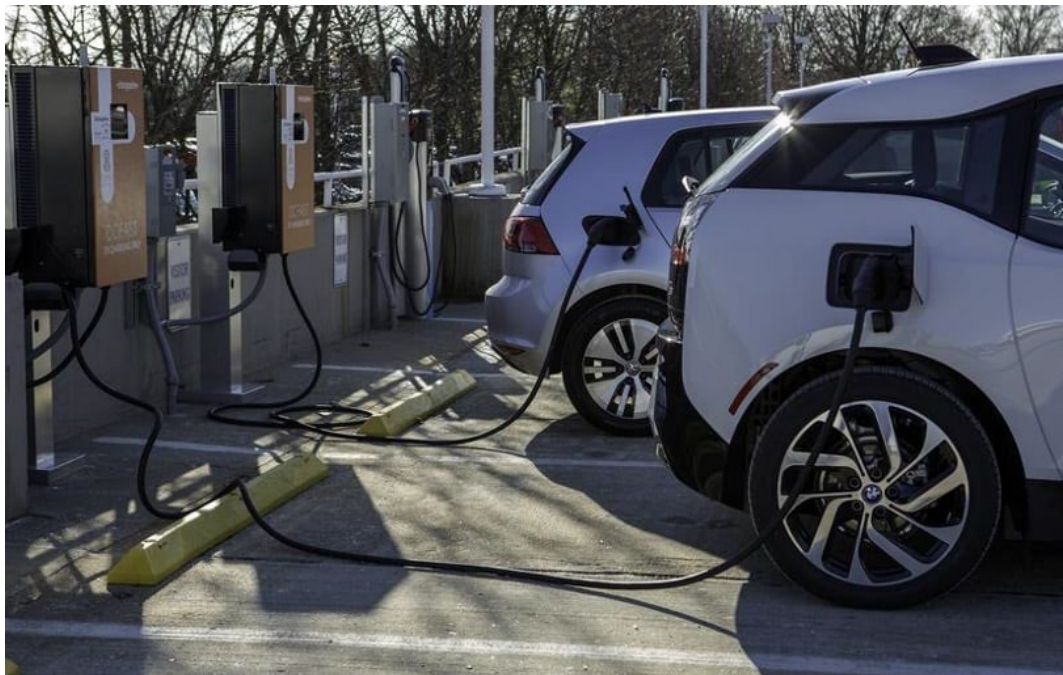
Figure 3 Level 2 Charging Infrastructure (Mlot, 2016)
