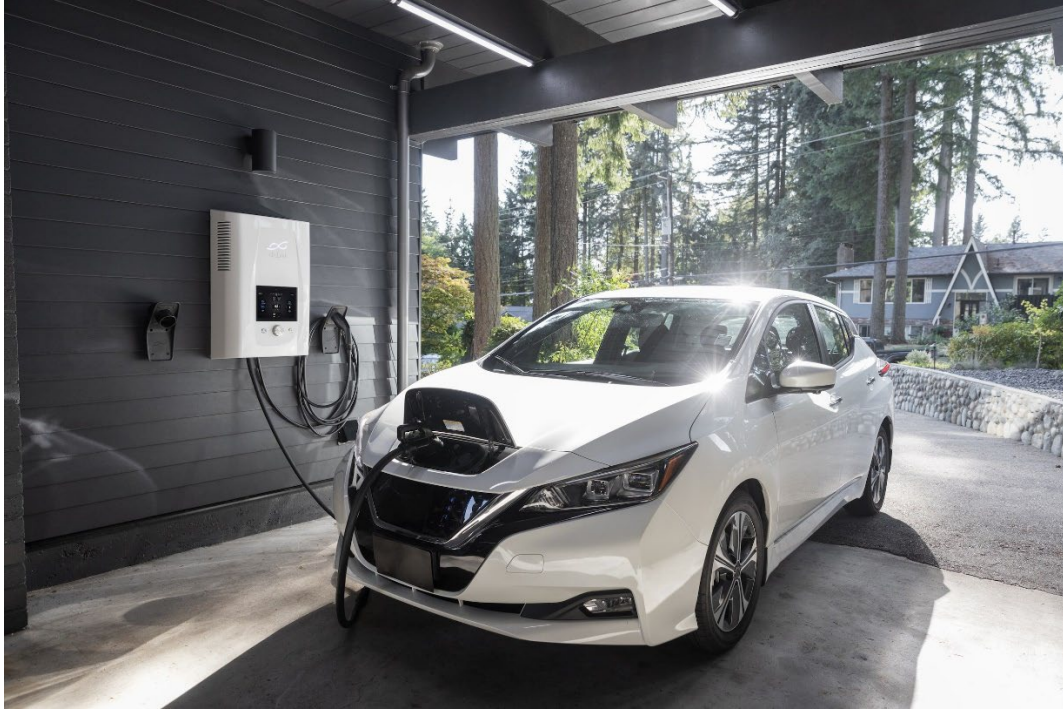
Figure 2 Level 1 Charging Infrastructure (Evenflow Home and Commercial Services, 2024)
