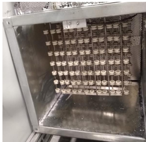
Figure 85: Two 4 kW Resistance Heaters Installed in Ducted Closed Loop
