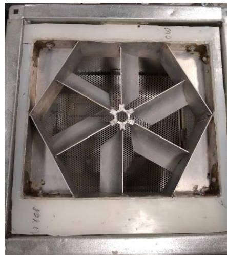
Figure 86: Air Mixer Installed Downstream of Heaters
