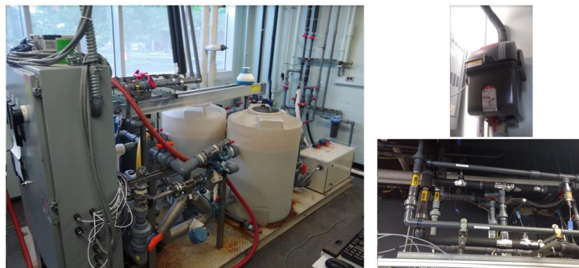
Figure 9: (Left) Hot and Cold Water Distribution Skid; (Top-Right) Honeywell Humidifier; (Bottom-Right) Water and Glycol Distribution Lines into Air-Loop's Conditioning Coils
