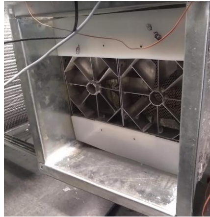
Figure 83: Air Mixers Installed at Air Supply Side
