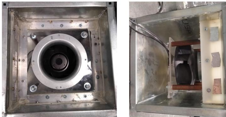
Figure 90: (Left) Centrifugal Fan Inlet (Right) Centrifugal Fan Outlet
