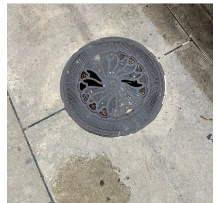
Figure 27: Photo showing clogged on site drain (Photo Cred: Kelly Rasmussen)
