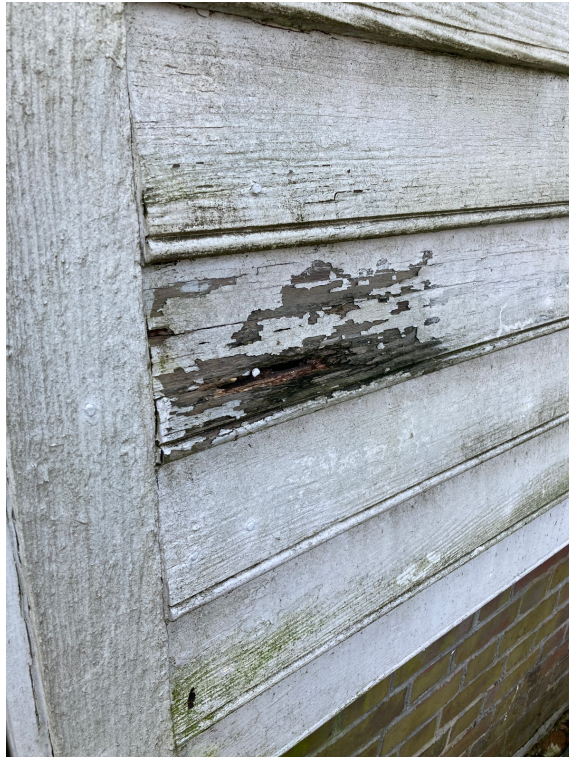
Figure 4.10 - Damage on weatherboarding (Photo by author, 2022).
