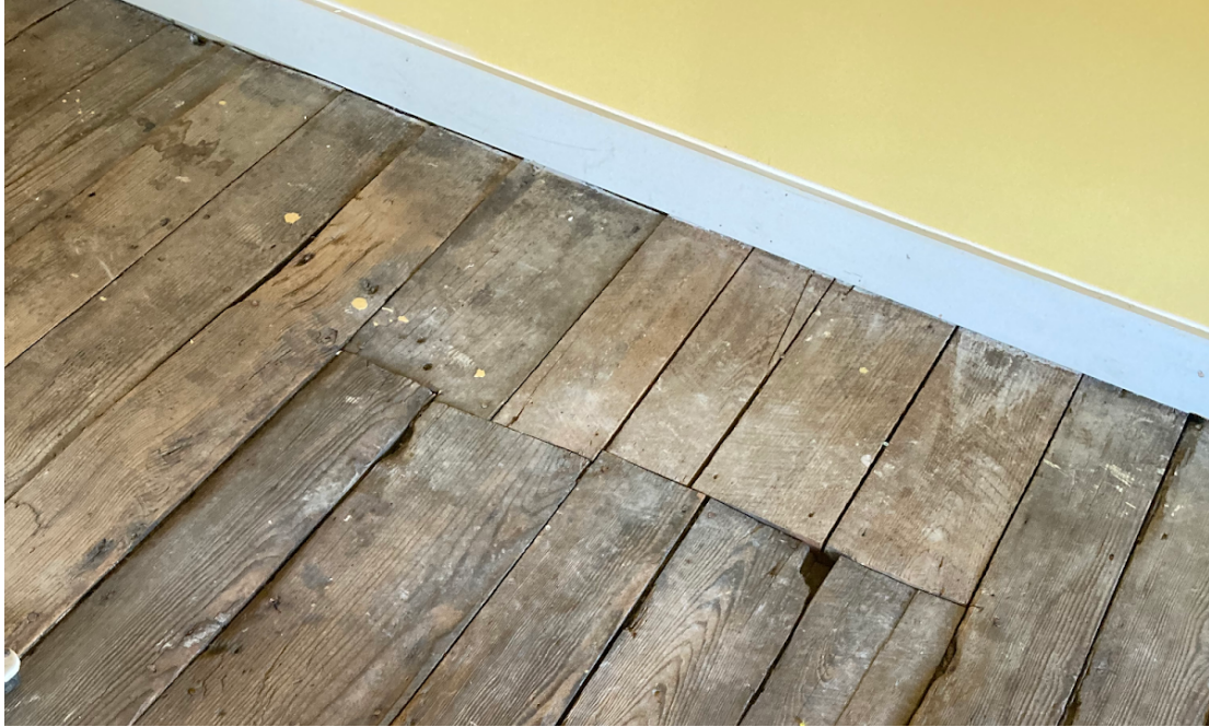
Figure 3.52. Attic in kitchen with repairs of circular sawn lumber. (Photo by author, 2022).
