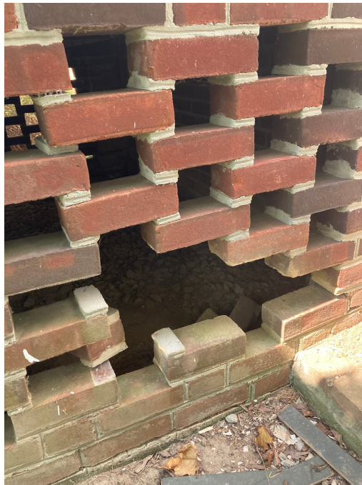
Figure 4.9. Damaged brick latticework on front porch (Photos by author, 2022).
