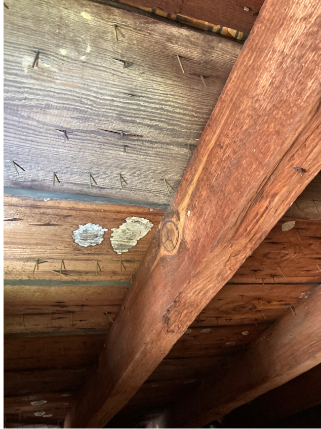
Figure 3.31. Cut and wire nails in attic decking (Photo by author, 2022).
