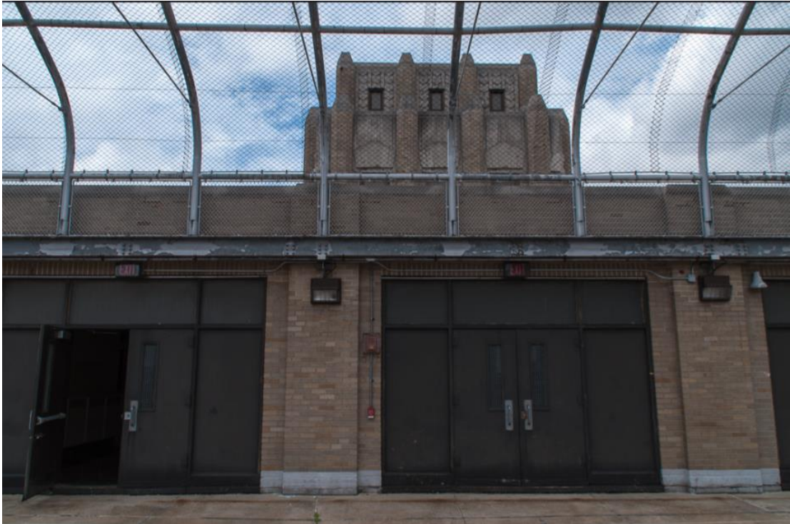
Figure 11. Vaux exterior deterioration in 2013 (Photo by Tieshka Smith).
