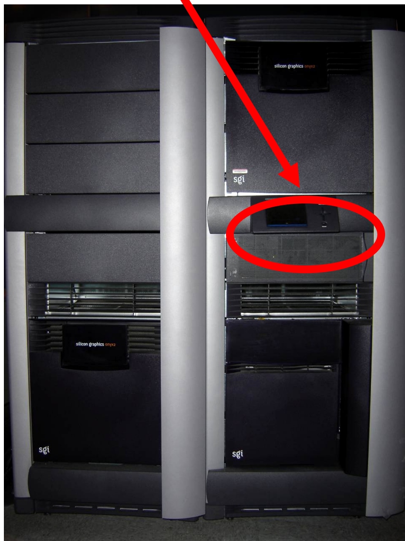
Figure 61: Onyx2 Main Panel Location
