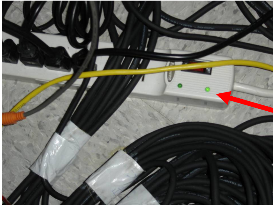
Figure 65: Power Strip Behind Huron PC
