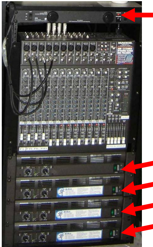
Figure 70: Switches for the Mixer and Amplifiers
