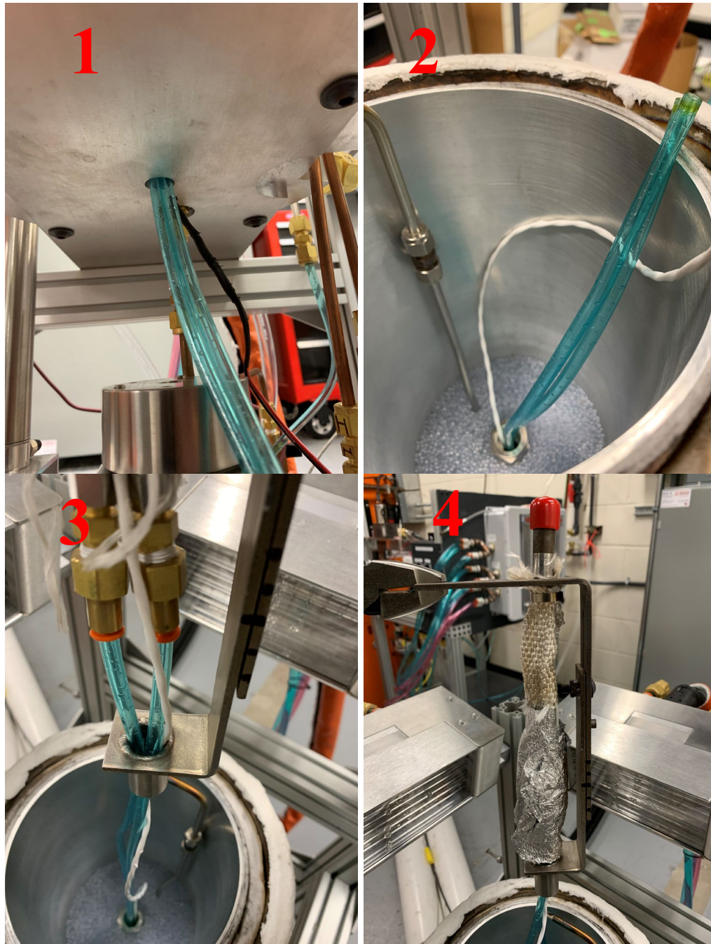
Figure B.17: The four stages of running the water lines into the heat flux gauge.
