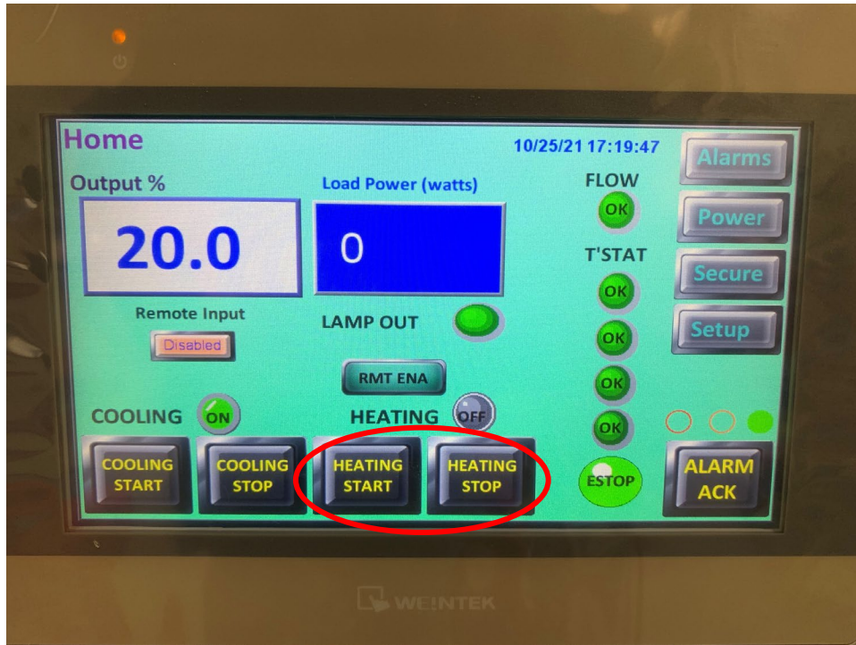
Figure B.10: Heater start and stop location on screen.
