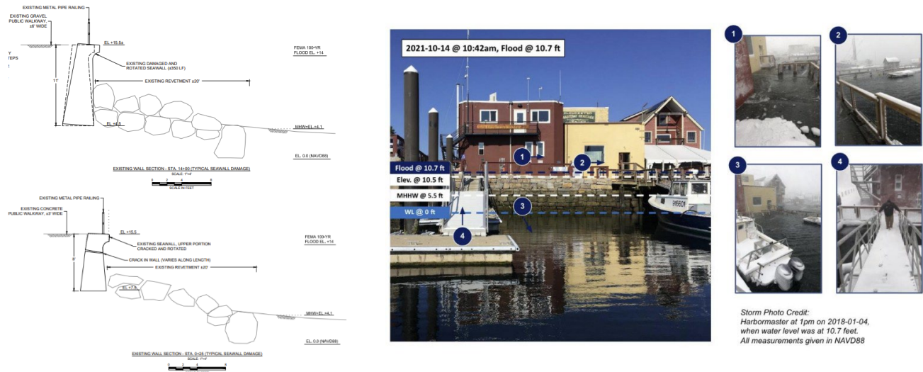
Figure 37: Existing seawall conditions and documented flooding during the 2018 storm surge event within the selected waterfront district in Gloucester, illustrating vulnerable edge conditions, storm surge impacts, and deterioration of waterfront infrastructure. Image source: City of Gloucester, 2025 Gloucester Municipal Harbor Plan and Designated Port Area Master Plan (2025).
