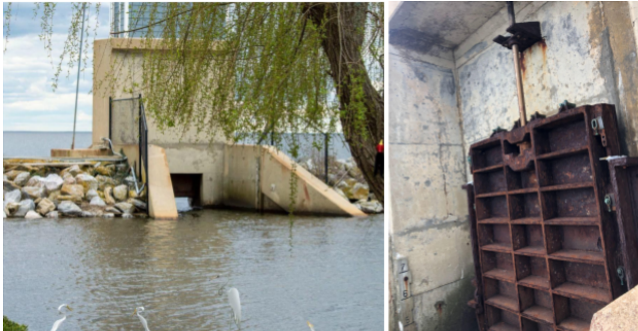
Figure 5. Current floodgate connecting Stinint's Marsh to Chesapeake Bay, shown fixed in the open position
