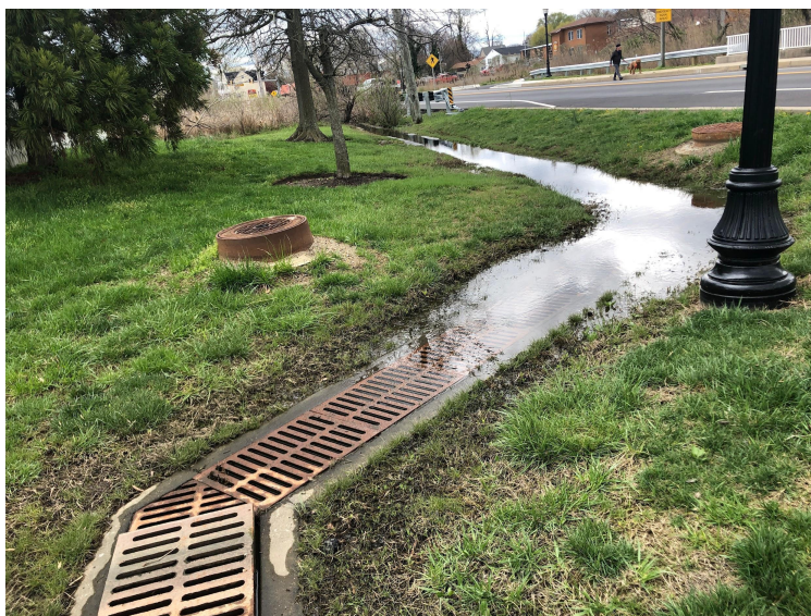
Figure 3. Seagate stormwater drainage system inundated during high tide (April 5th, 2024)
