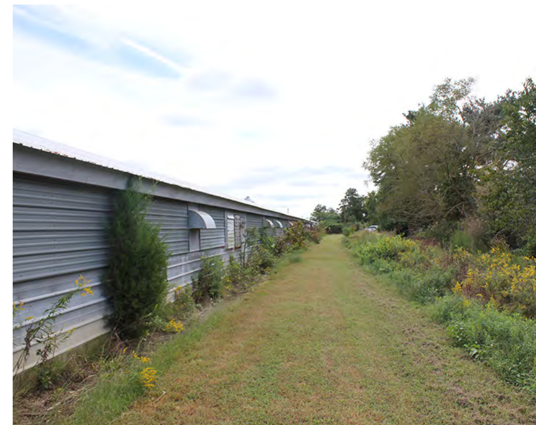
CLOCKWISE FROM TOP: 52,740 sf of corrugated galvanized steel is available from existing chicken sheds on site; Additional view of chicken shed on site; Existing grain silos on site may be re-purposed
