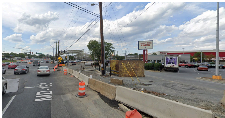
Fig 56. There is a gap in the sidewalk on the north side of University Blvd approaching the New Hampshire Ave intersection due to Purple Line construction.
