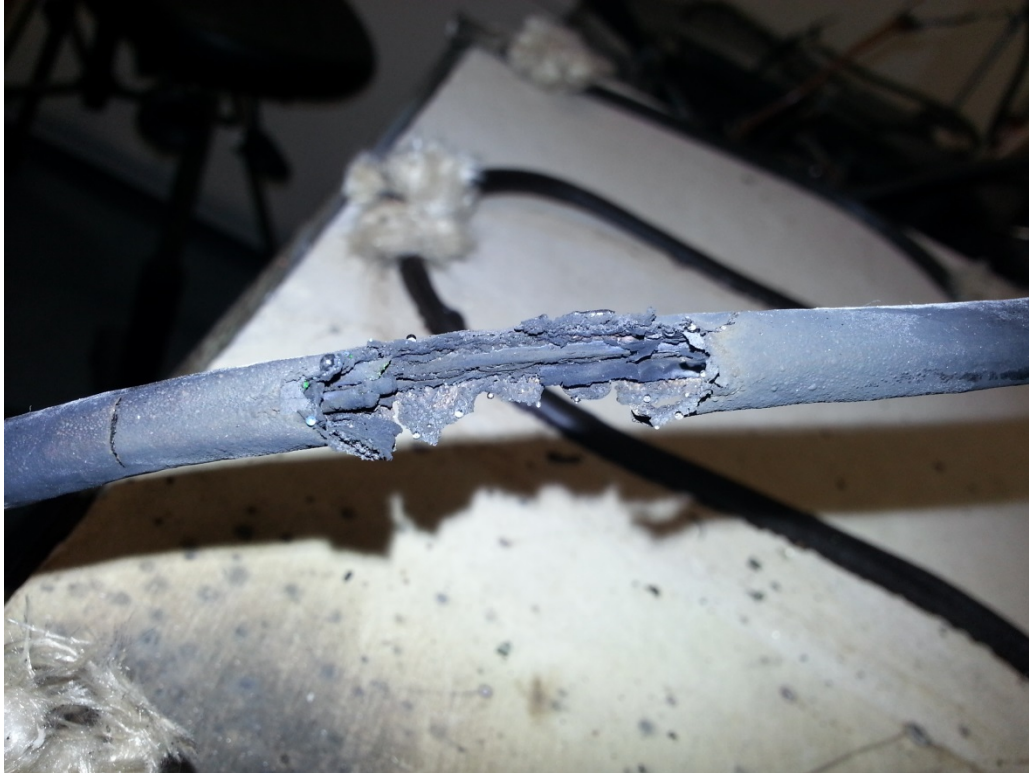
Figure 47: Post Arc Failure (Destroyed hot and ground wires)
