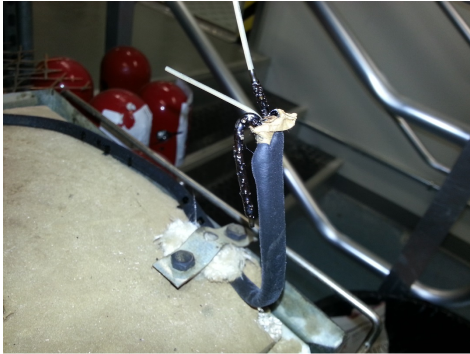
Figure 43: Bubbled, Cracked Inner Insulation (Post Exposure)
