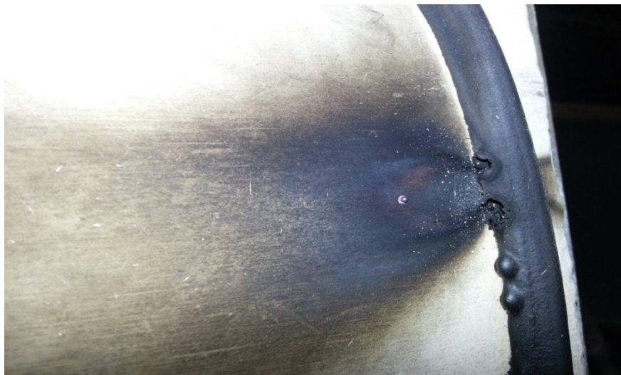
Figure 11: Cable Arc Aftermath
