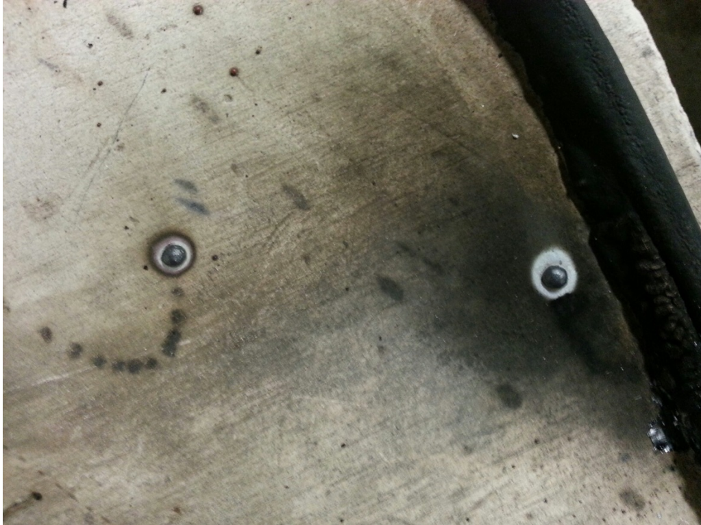
Figure 49: Copper Beads Ejected From Cable During Arc Failure
