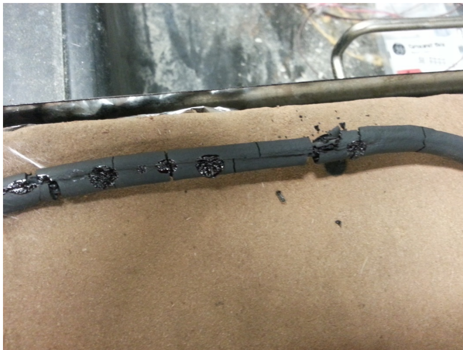
Figure 44: Bubbled, Cracked Outer Insulation (Post Exposure)
