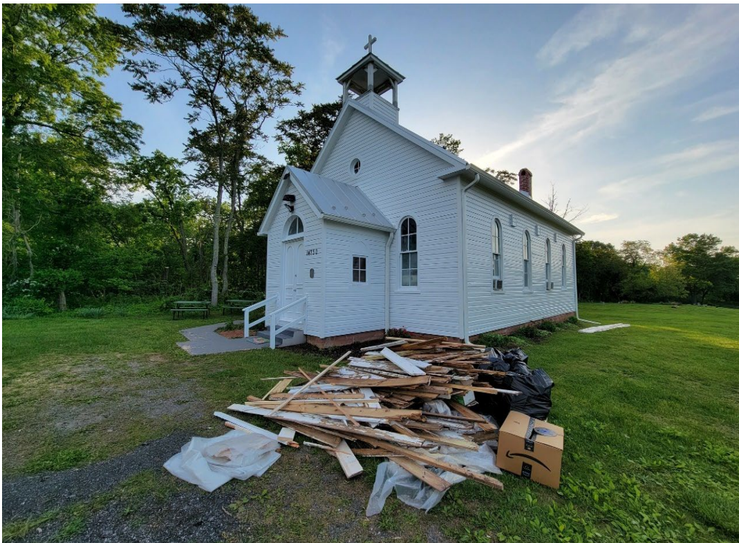
Figure 9: Restoration efforts taking place at St. Paul Community Church in Sugarland (SEHP Facebook, 2023).
