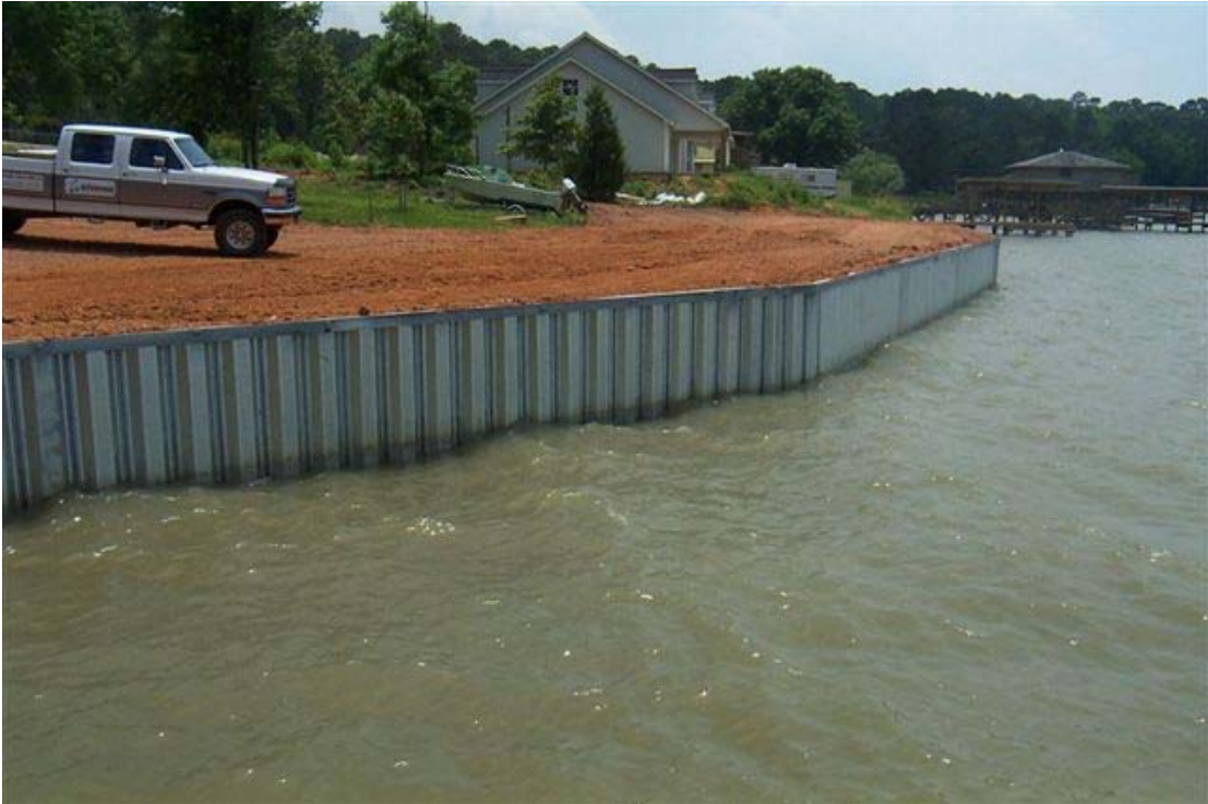
Figure 9. Steel bulkhead along a new shoreline development. Image taken from Waterside Construction website: http://www.watersideconstruction.com/Waterside%20Construction%20Bulkheads.htm
