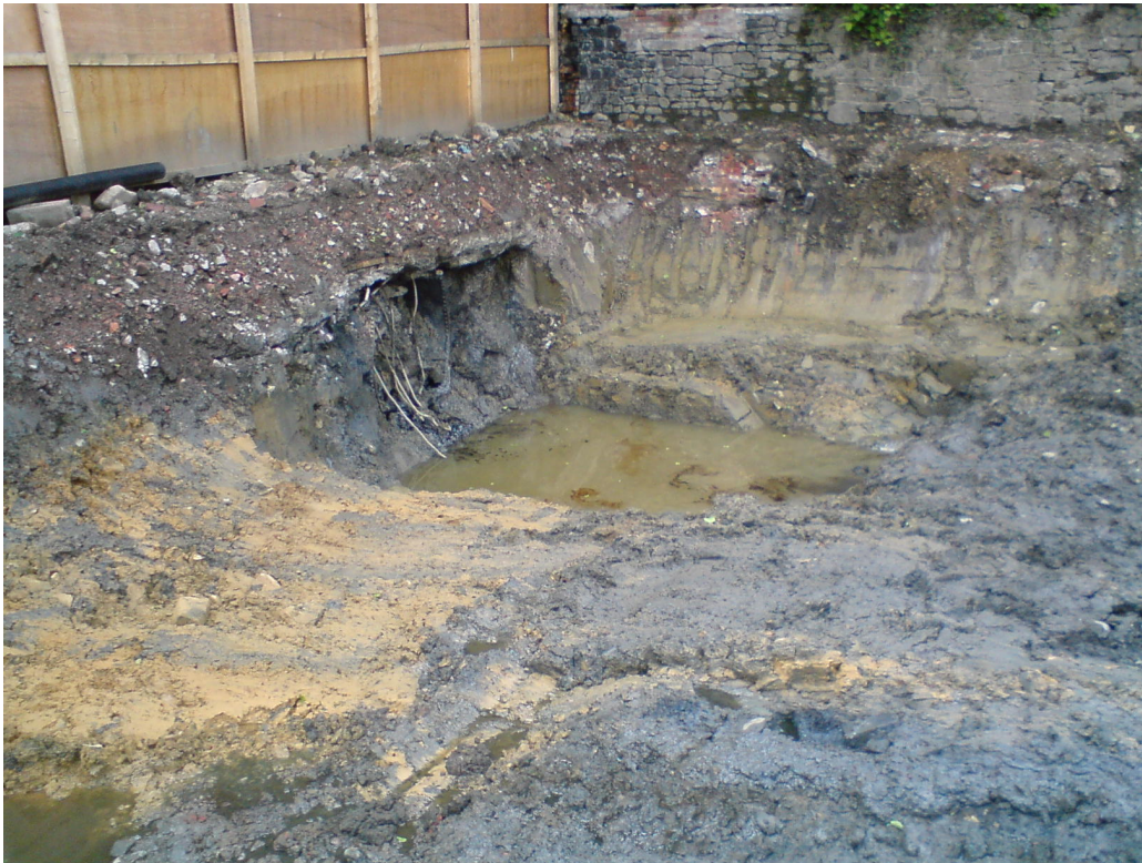
Figure 28: Soil contamination caused by underground storage tanks containing tar. Encountered during remediation works at a disused gasworks. (Source: Dumelow)
