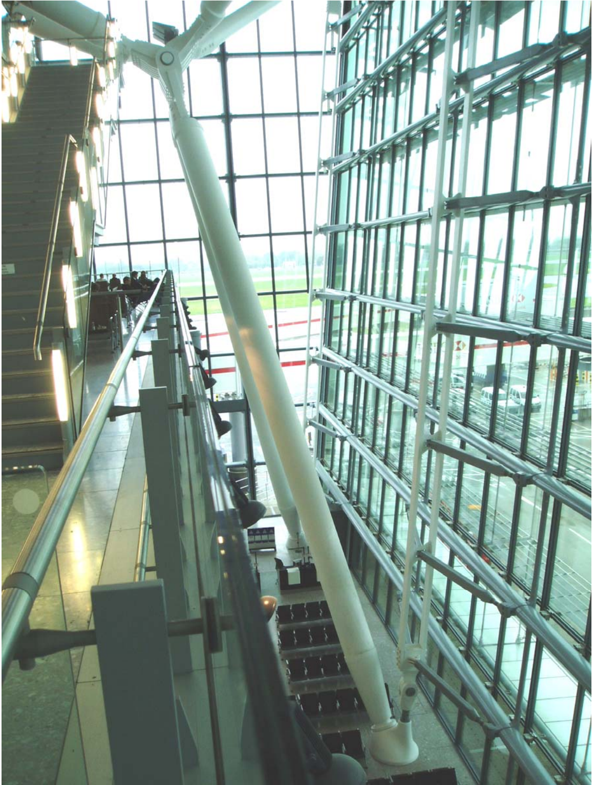
Figure: I-2 – Heathrow Airport Terminal 5. Designed by Richard Rogers Partnership. Structural column to roof and curtain wall detail. Personal photo taken May 2008.
