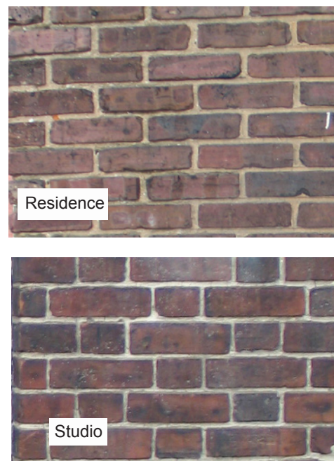
Figure 16. Residence brick (running bond) is uneven with thicker mortar joints, while the studio brick (Flemish bond) is more refined with thin mortar joints (Author)
