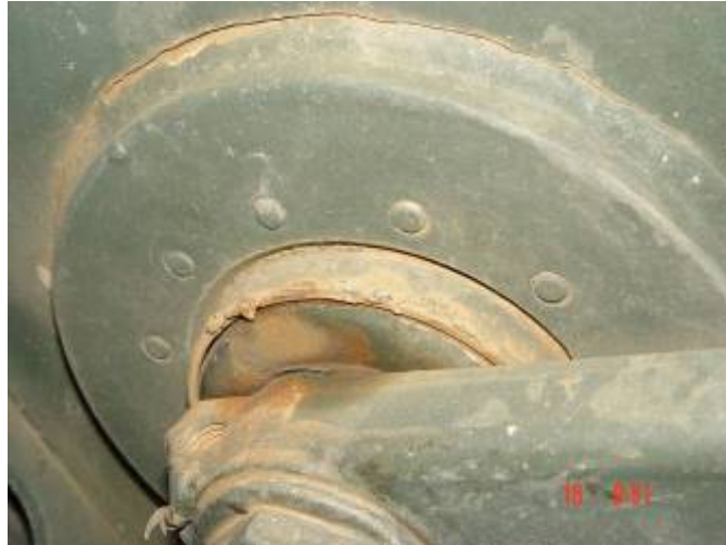
Figure 4.2: Example component with fatigue crack
