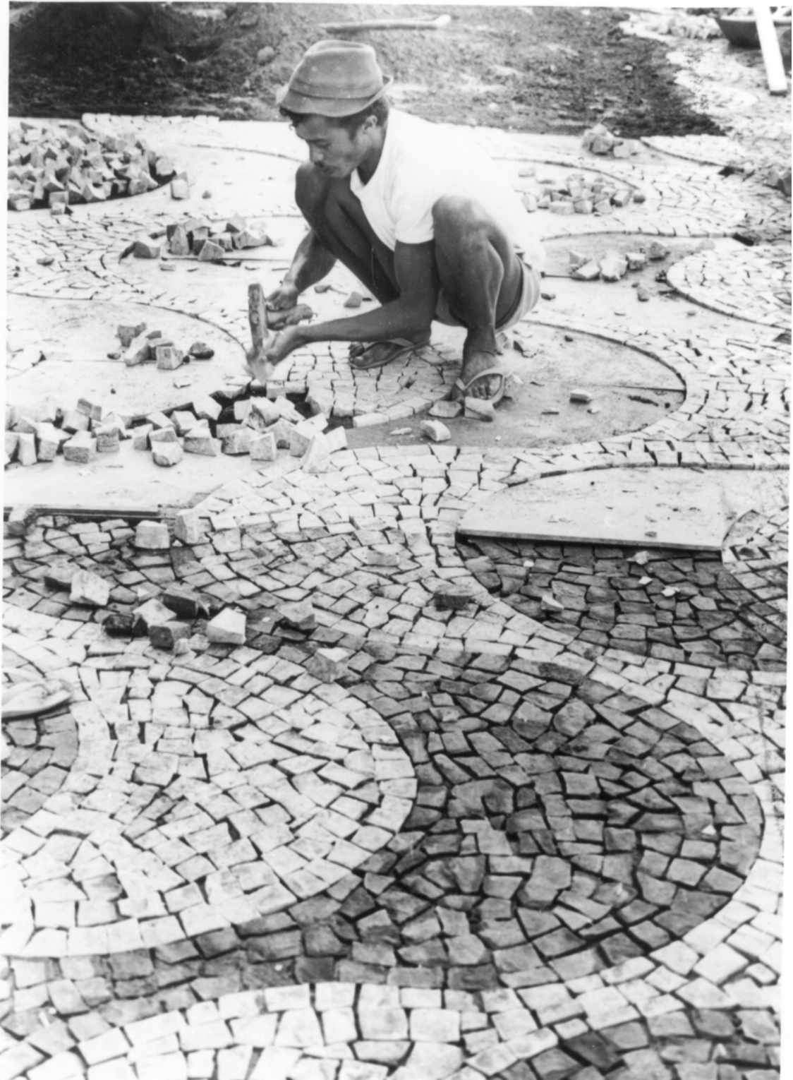
Figure 5.10 Work on Roberto Burle Marx's famed sidewalks along the new Avenida Atlântica
