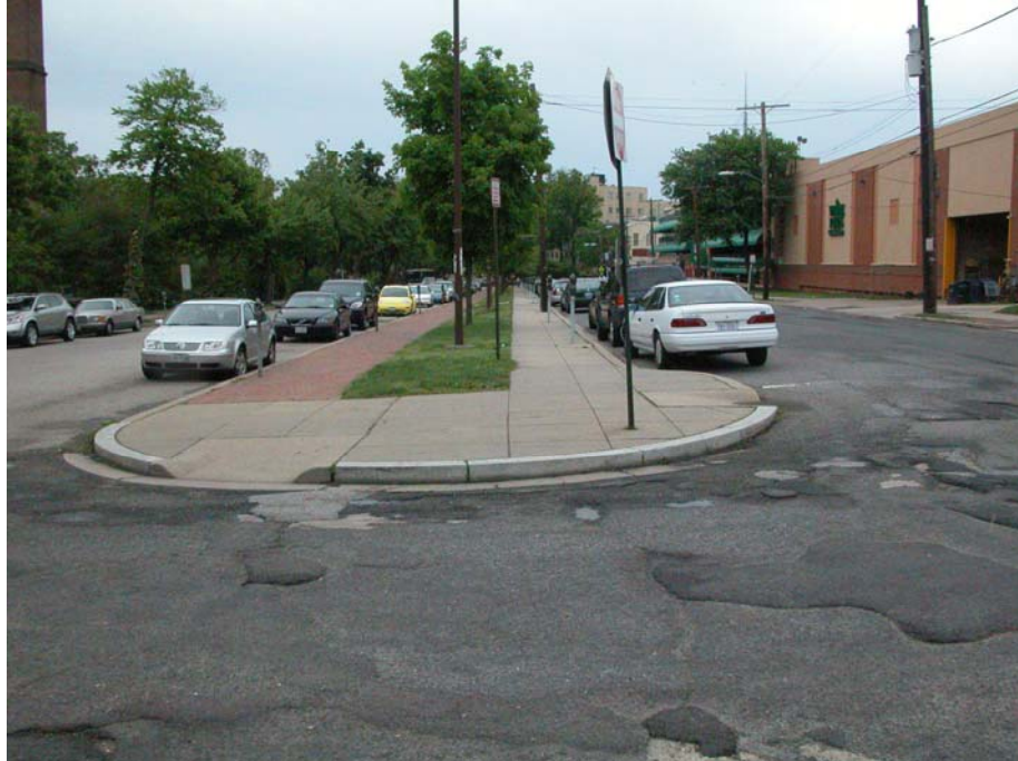
Figure 24: View of Median Strip between Fort Reno Drive and 41 st –the site is located on the right of the picture.
