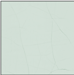
GROUT COLOR MINOR WORN TEXTURE
