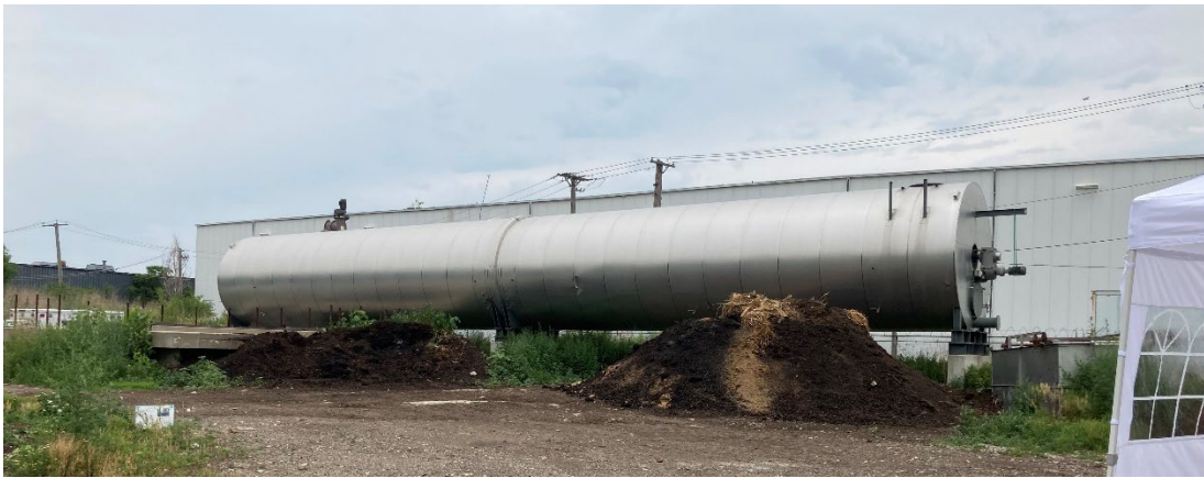
Figure 68: The anaerobic digester at The Plant in Chicago, IL.
