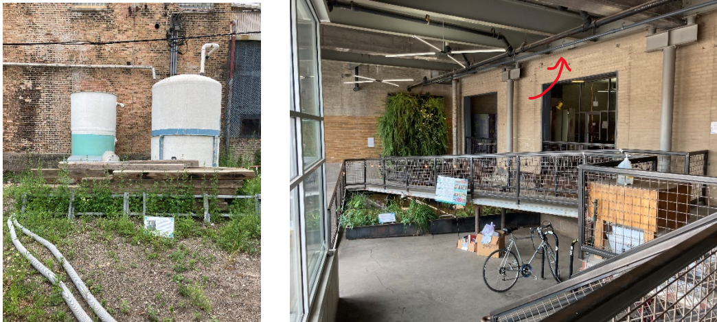
Figure 69: Rainwater capture and carbon dioxide capture and reuse put into practice at The Plant. Left: Rainwater capture systems feed underground cisterns that hold 9000 gallons of water. Right: Shown are the grey CO 2 lines that run throughout the building, supplying the excess CO 2 from The Whiner Brewery to use in the indoor farms.
