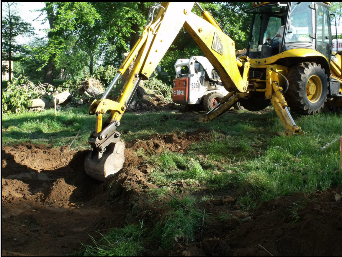
Figure 13: Photograph depicting the grading of the APE during the planned driveway re-routing.
