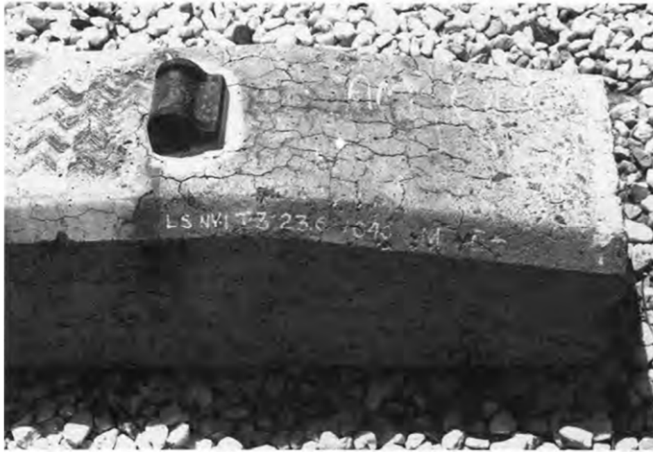
Figure 1.1: Precast, Prestressed Railway Tie Showing Signs of DEF-Induced Cracking
