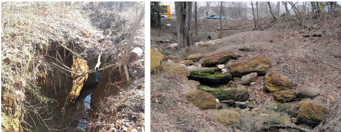
Figure 12. Eroded outfall RSC before (left) and after (right) restoration (Underwood & Associates)
