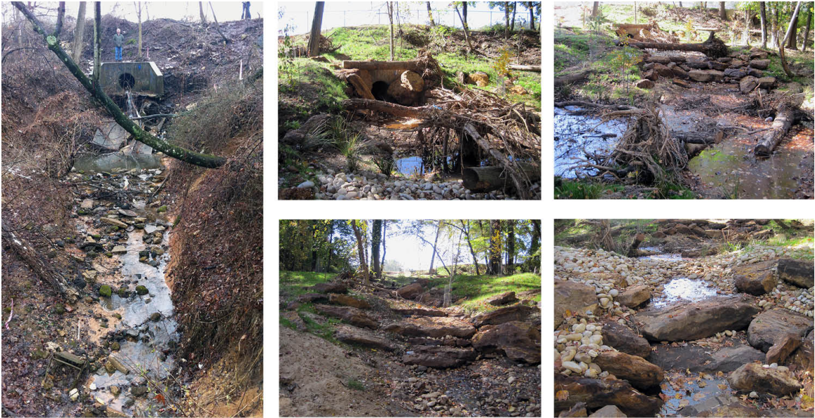
Figure 15. Brier Mill Run RSC before (left) and after (right) restoration (Biohabitats, left, and the author)
