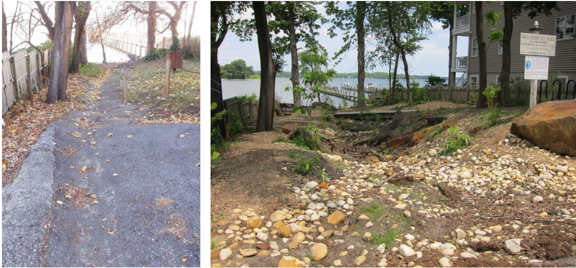
Figure 16. Cypress Beach RSC before (left) and after (right) restoration (Anne Arundel County Department of Public Works)
