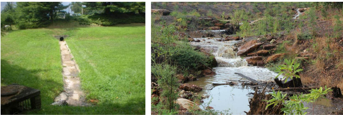
Figure 13. Upland stormwater retrofit RSC before (left) and after (right) restoration (Underwood & Associates)
