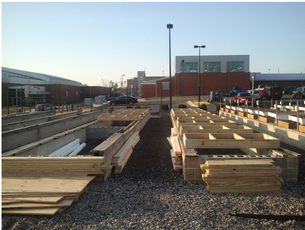
Fig. 5.1. Photograph of construction of the experimental green roof platforms at the Research Greenhouse Complex at the University of Maryland, College Park in May 2012.
