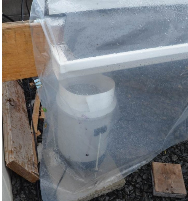
Fig. 5.4. Photograph illustrating a TB-4 rain gauge installed on one of the sixteen experimental platforms.
