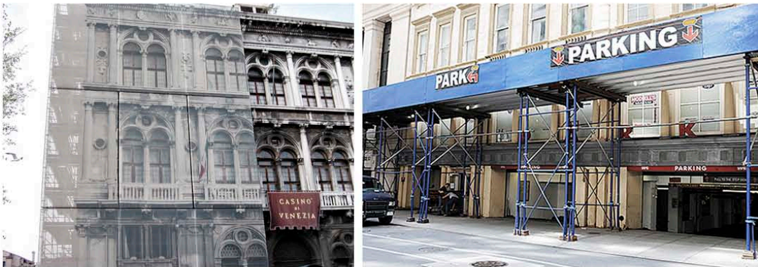
Figure 24 Artificial and temporary skinning through the construction process in Venice vs. basic scaffolding system creating a new space [images provided by author]
