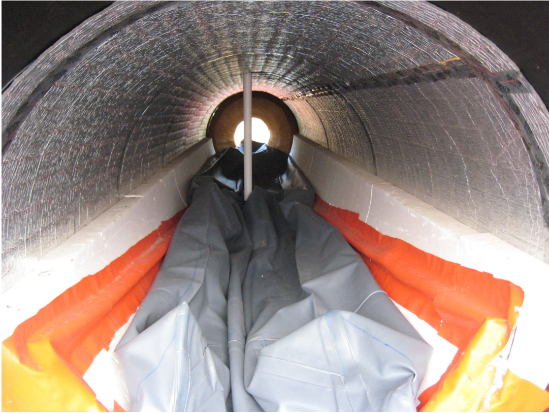
Figure 2-2 – The Maryland PVC bag digester with insulation. Pictured is the 2” EPS foam “nest” (white), the PEX hot water piping (orange), the PVC biodigester bag (gray), the radiant barrier (silver material on ceiling of culvert), and the biogas port (white PVC pipe).
