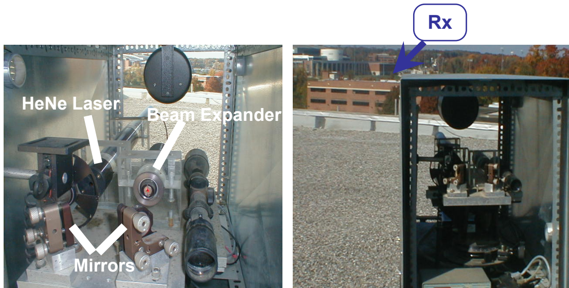
Fig. 3.2: Transmitter of the 863m link from AVW to Chesapeake Building.
