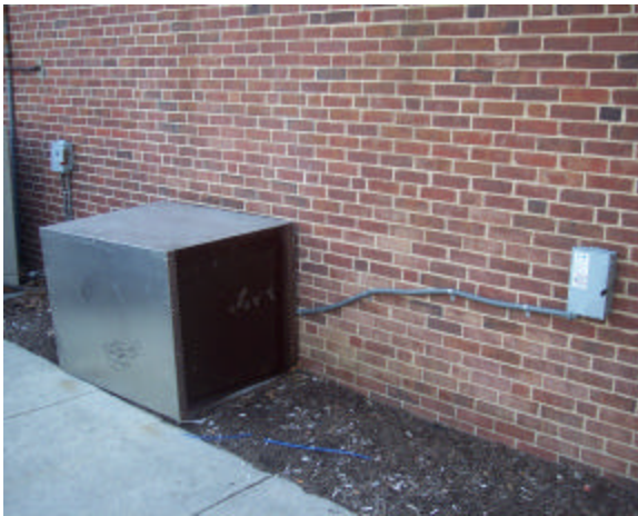
Figure 5 – Condensing Unit and Electrical Disconnect
