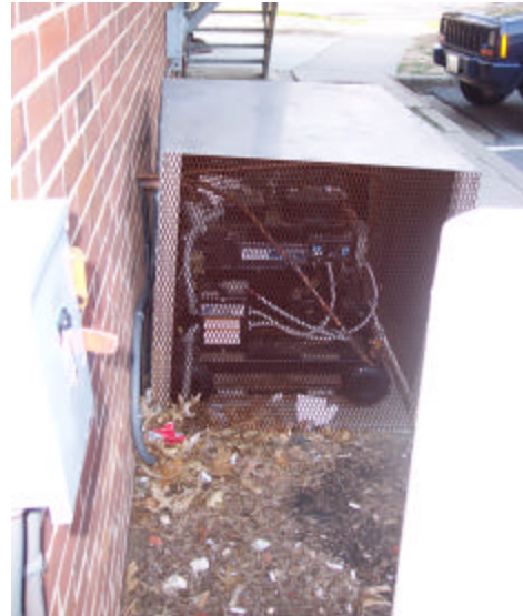
Figure 6 – Condensing Unit and Cover
