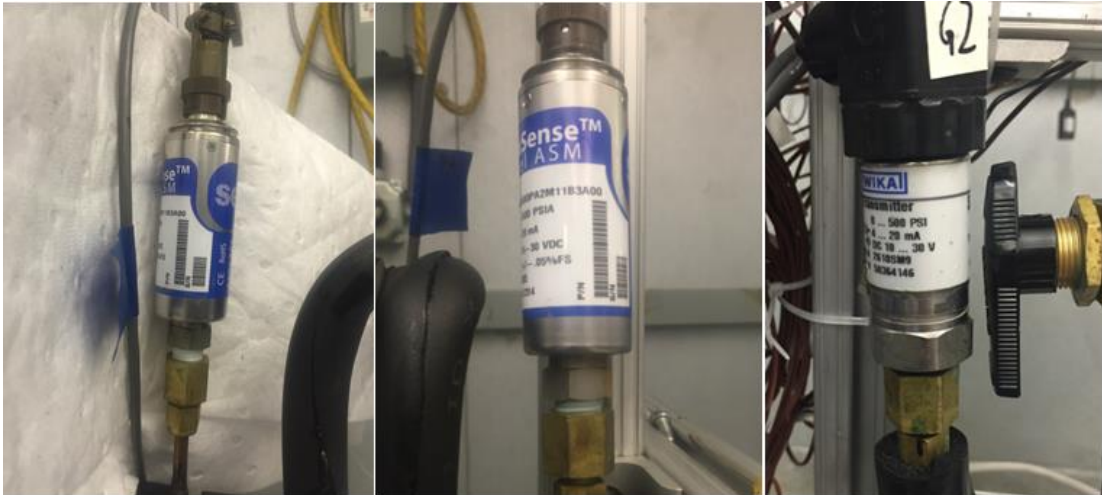
Figure 13: Pressure transducers installed in system (Left: Setra pressure transducer at evaporator outlet; middle: Setra pressure transducer at expansion valve inlet; right: Omega pressure transmitter at compressor discharge)
