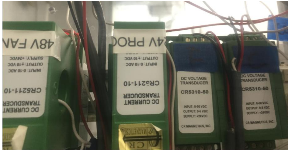
Figure 23: DC current and voltage transducers
