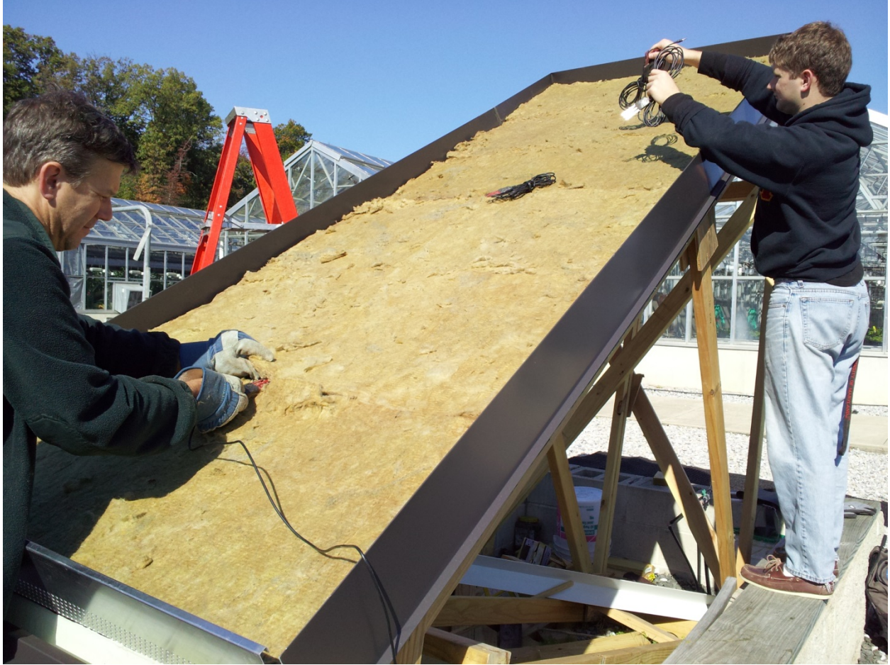
Figure 34. Installing probes on 45 degree module after laying out rock wool layer. Taken in Oct. 2013 (Courtesy of Ben Borchers)
