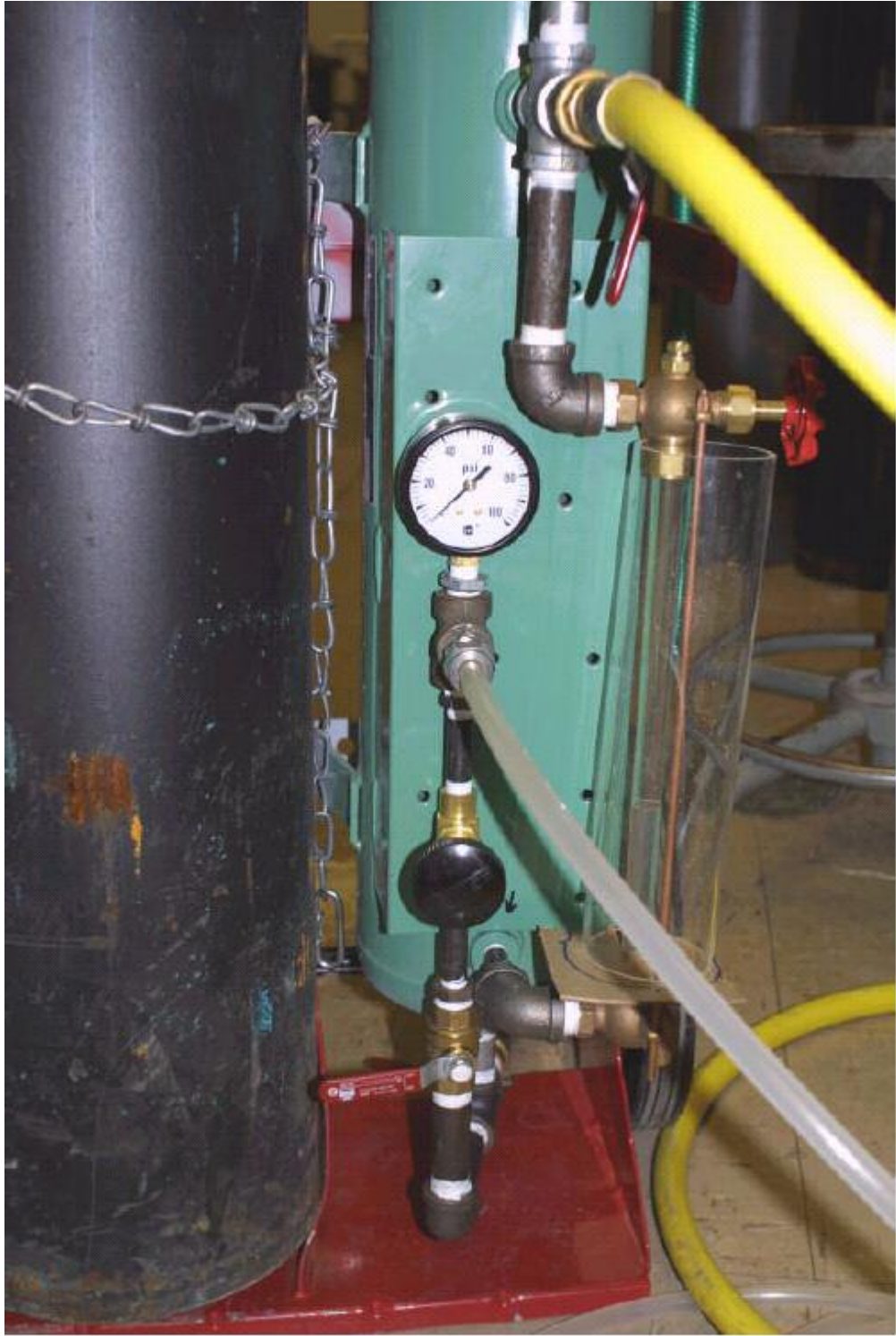
Figure 6: Solution Tank, Level Gauge and Connections
