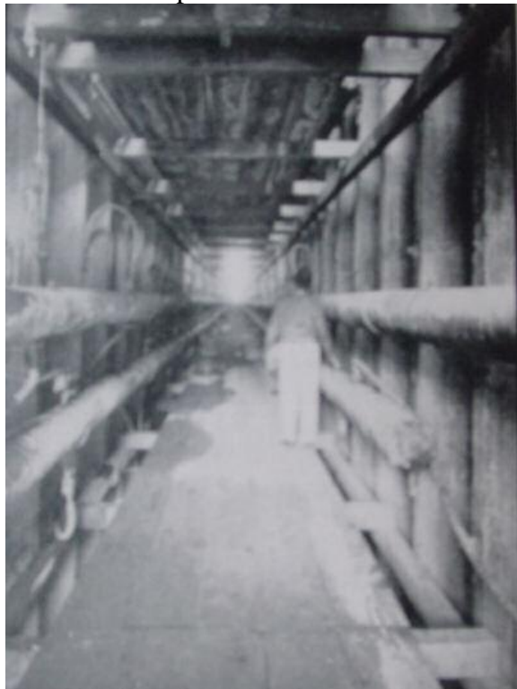
Plate 13 Walkway through the Hoover dam with supply lines for cooling pipes.
