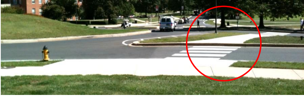
Figure 14 Missing ADA facilities near “Big M” roundabout.
