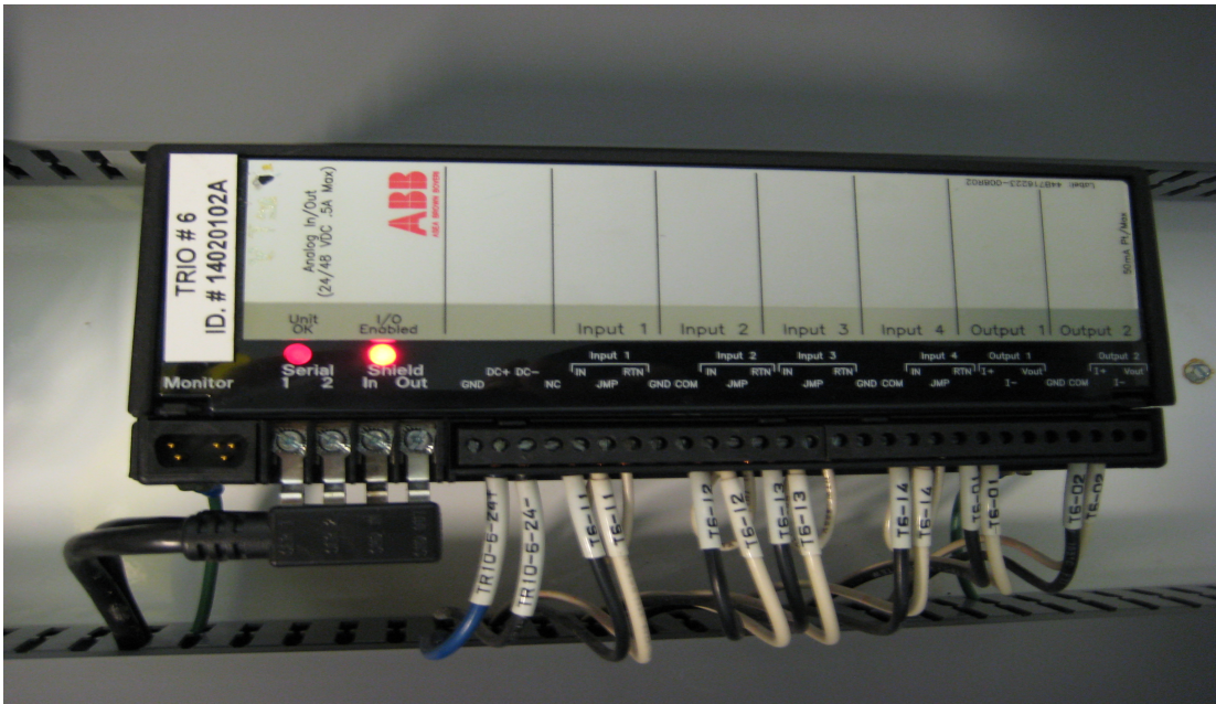
Figure 1.3: Trio block used make DCS connections to histidine weighing scale, pH transmitter and the pump
