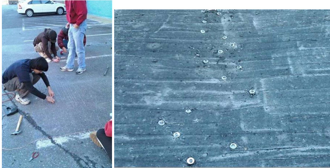
Figure 15. Placing wires on the parking space before covering with sealant (left). Masonry nails were used to hold the Nichrome wires on the pavement (right).
