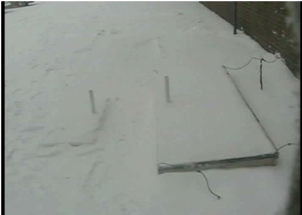
Figure 32. The SnowMelt system with fresh snowfall on the sealant before being switched on
